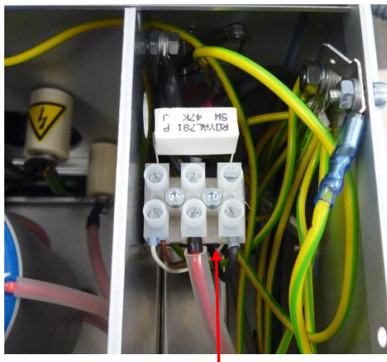
Ground sensor OFF (factory made)
